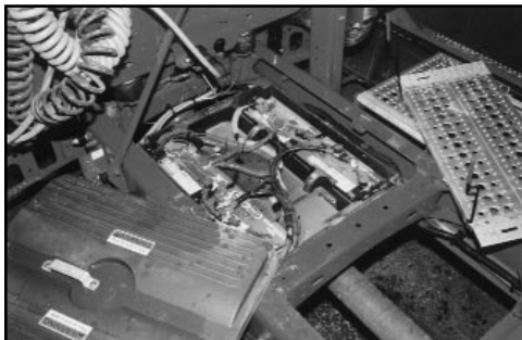
Columbia: battery box with cover removed
